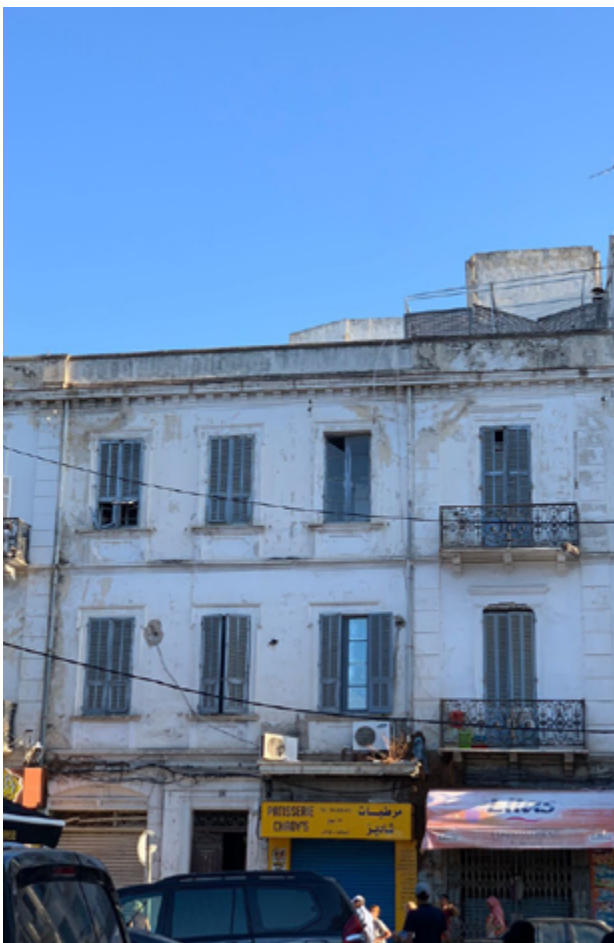
Figure 3.12: Photo of a neglected building taken from Al Jazira Street © Authors, 2024
