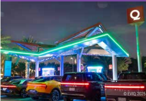
Figure 4.87: EVIQ's first public DC fast-charging site in ROSHN, Riyadh.
