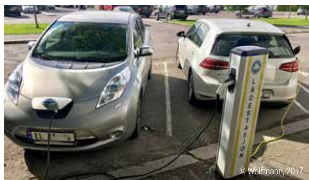
Figure 2.5: EV charging station in Storgata, Norway.
